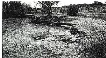
Slumping area at Murrayview
