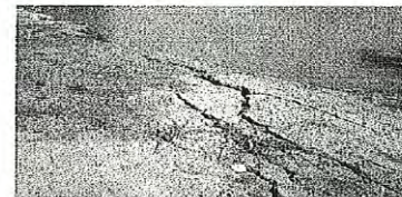
Riverbank cracking at Murrayview
