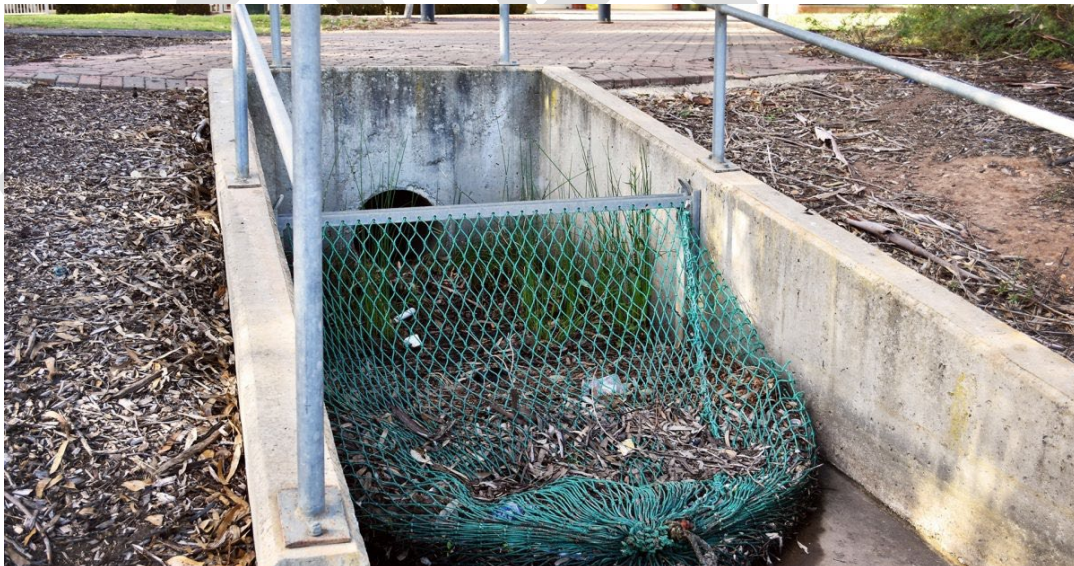
Figure 4: Trash rack to collect debris and rubbish in drain, uncleared can increase the risk of flooding during high rainfall events
