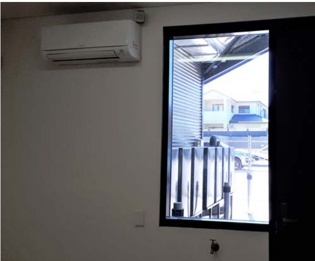
Figure 7: Details of the City of Burnside’s short-term holding facility, air-conditioning system
